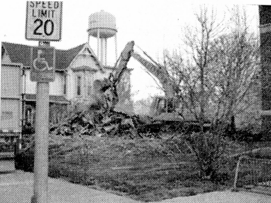
Jackson Demolition Services took down the former doctor's building on Kewanna's Main Street over the weekend to make room for the expansion of the Kewanna-Union Township Public Library.
