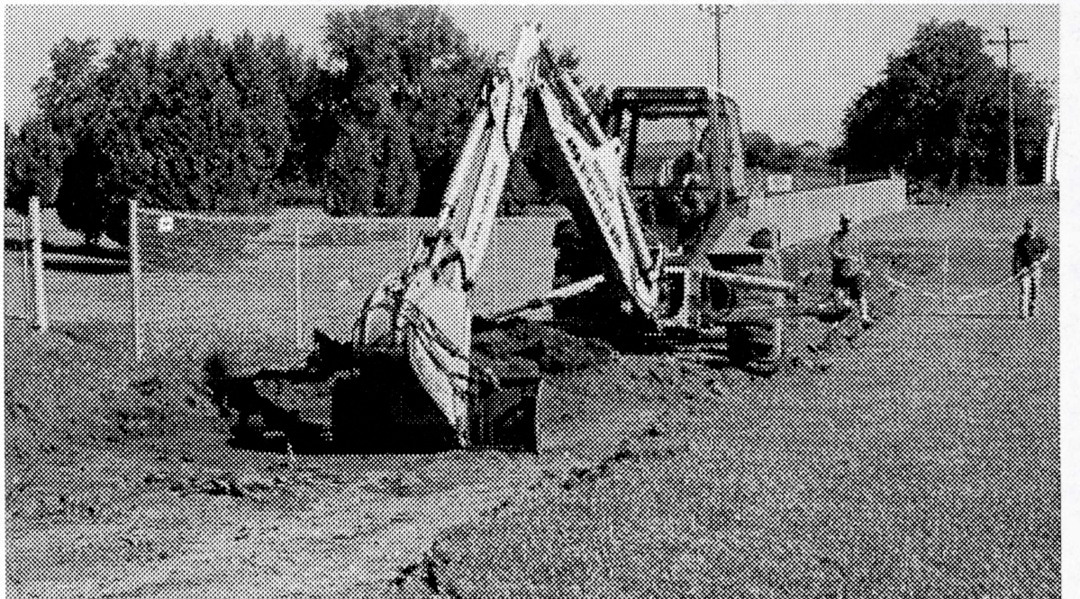
CONSTRUCTION UNDERWAY - Work began this week on the construction of a garden tractor pull track for this year's Kewanna Fall Festival. The festival runs September 26th, 27th, and 28th.
